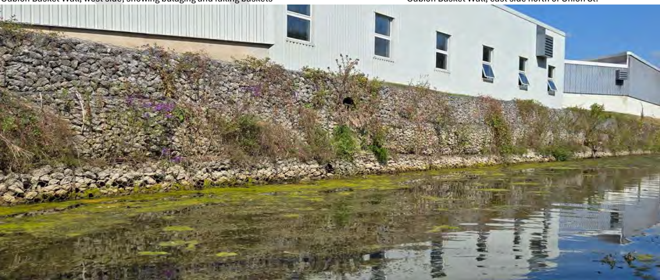
Gabion Basket Wall, looking north along west side of the river, north of Union St.
