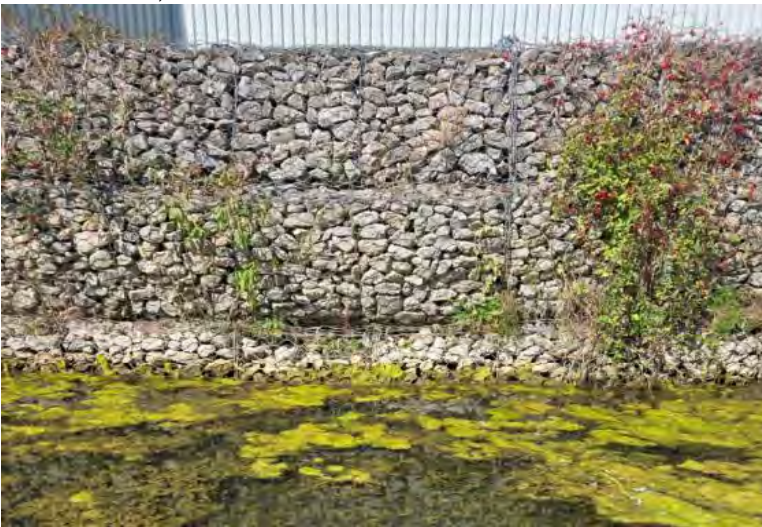
Gabion Basket Wall, west side, showing bulding and failing baskets
