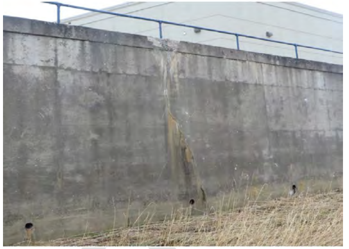
Showing a crack in the wall, allow water penetrate through the wall
