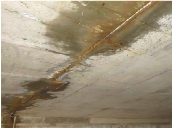
Example of construction joint leaking
