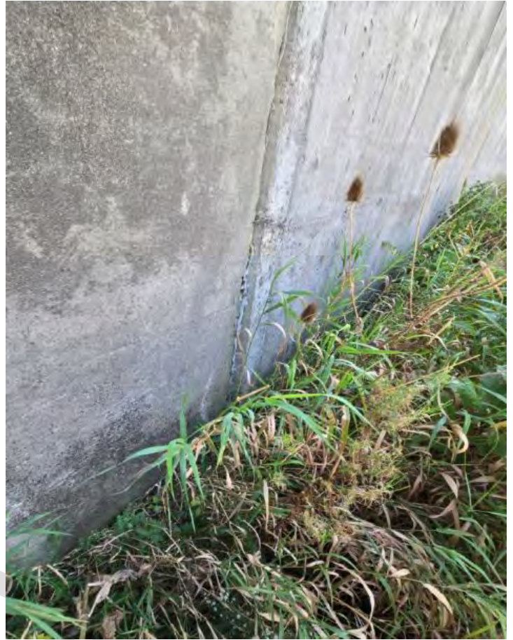
Retaining wall near the base of the wall where leaning out
