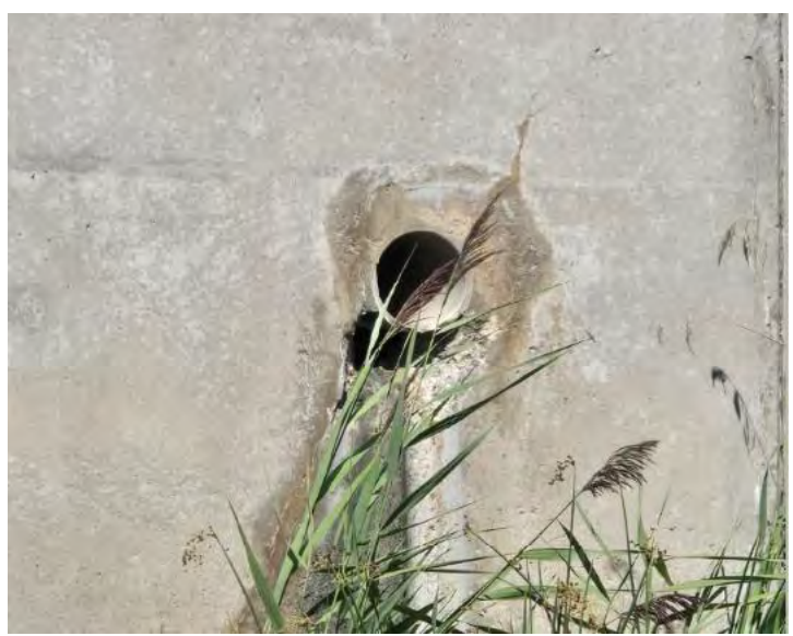
Example of typical drainage pipe through wall, and holes around pipe
