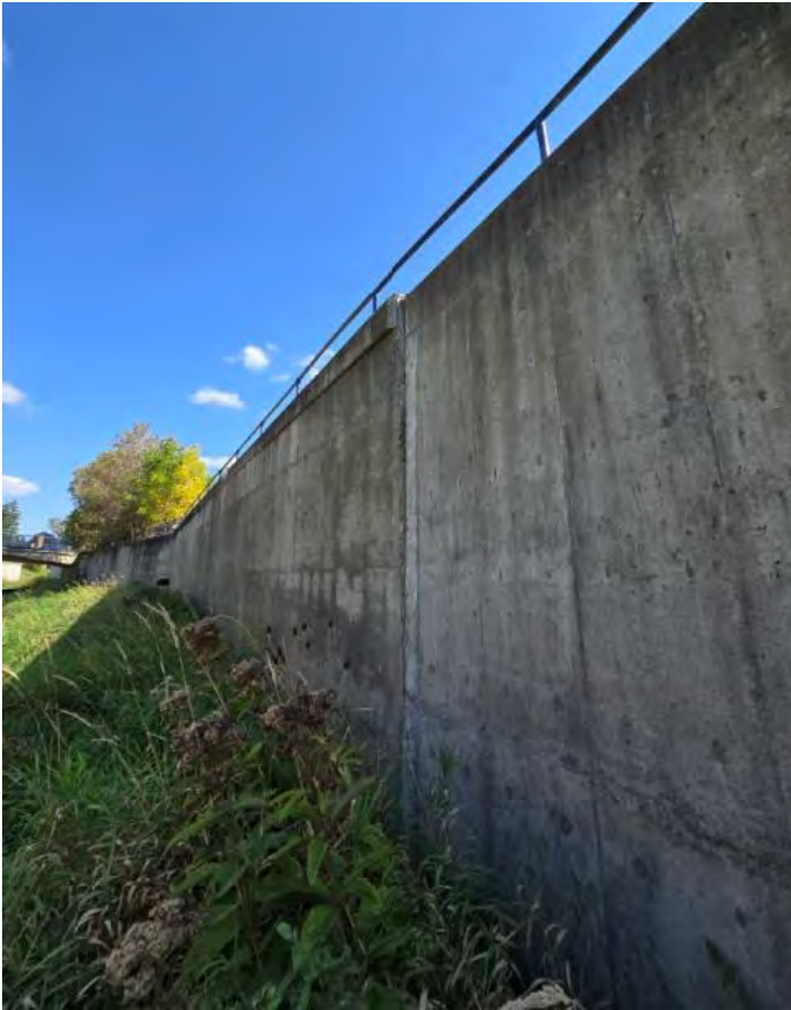
Retaining wall, showing top leaning out, looking north
