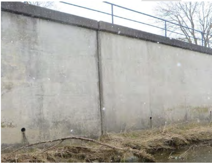
Retaining wall at north limits of section leaning outward
