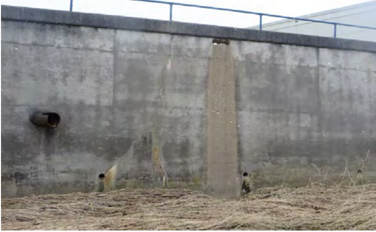
Showing where holes were drilled in the wall to let surface water through
