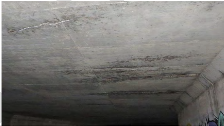
Example of cracks mid-way in culvert letting water penetrate top slab.
