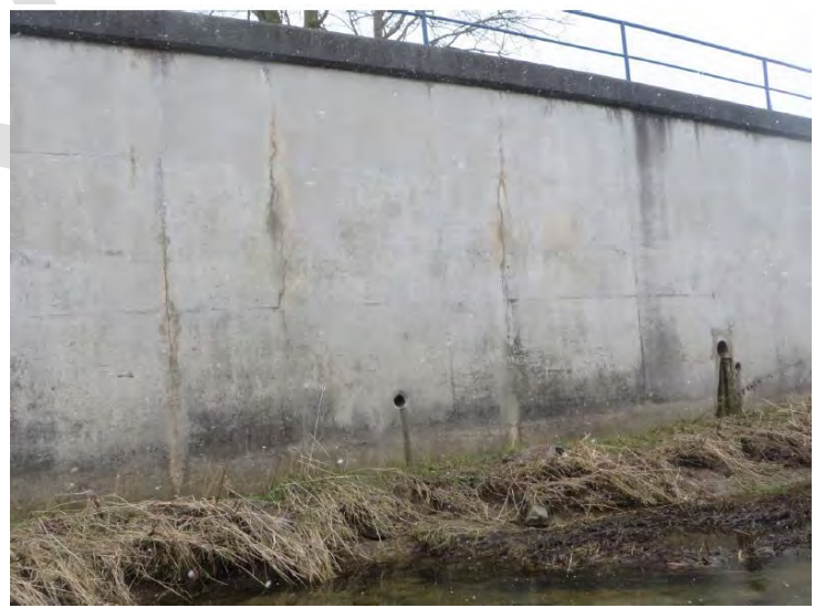
Retaining wall showing typical vertical cracks in the wall
