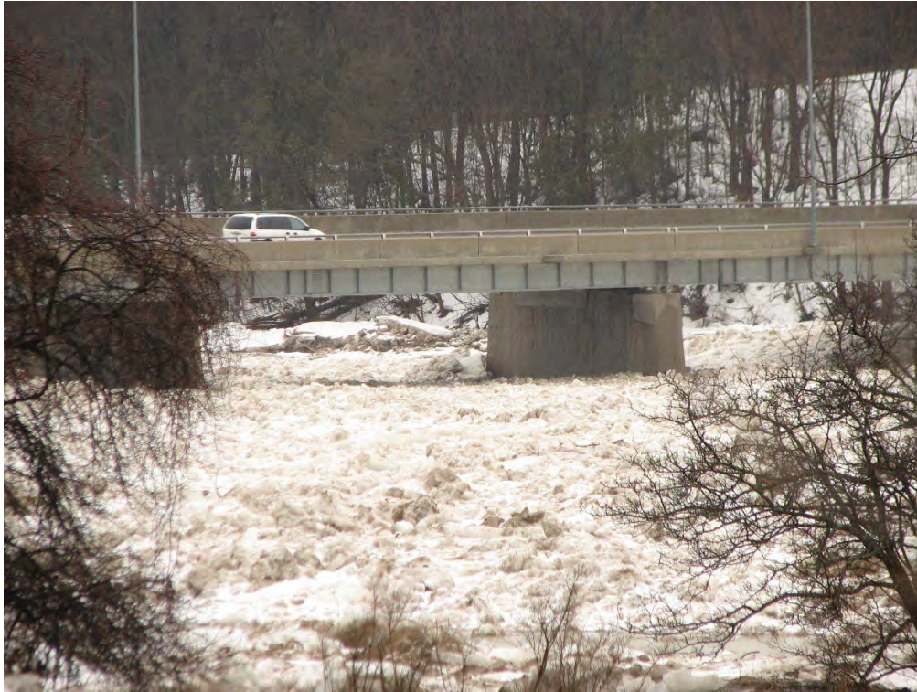
Ice build up surrounding the Highway 21 bridge in 2011
